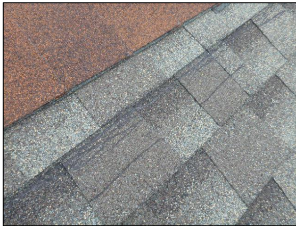
Horizontal creases in wind-damaged shingles.
